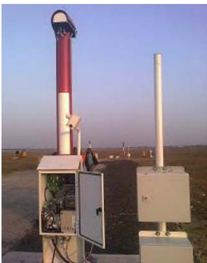
Fig. 16 Drishti at Runway 28 of IGI airport, New Delhi installed in January 2013.
